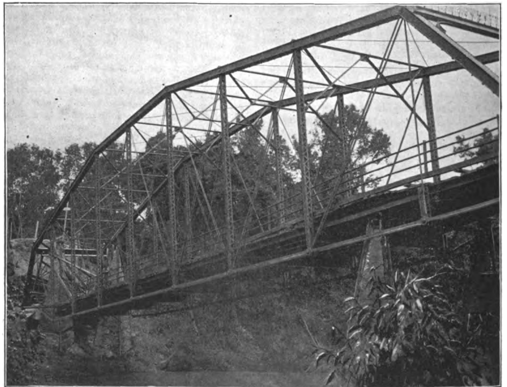
FIG. 1. GENERAL VIEW OF WRECKED BRIDGE OVER COLORADO RIVER AT GONZALES, TEX.
